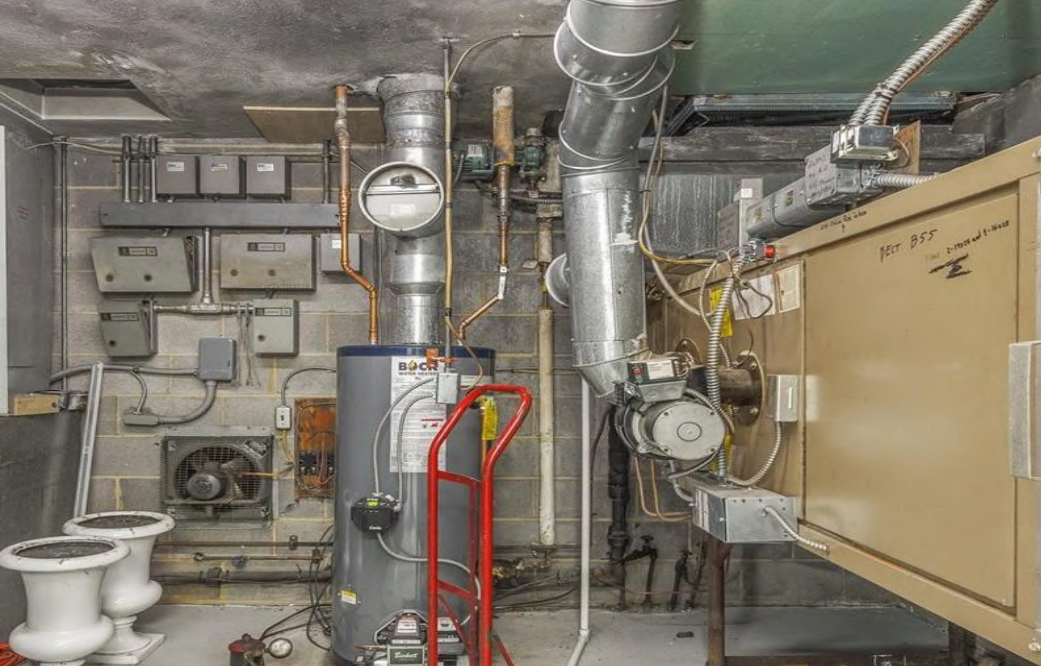
Hot Water Heater
