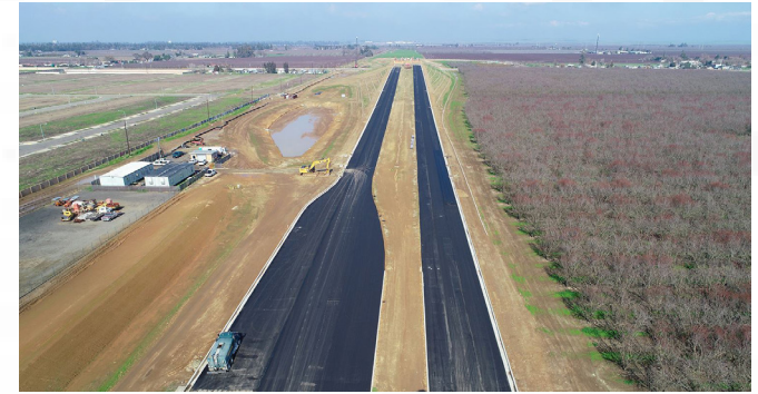
Campus Parkway Segment II, looking north toward U.C. Merced on the horizon (January 2019)
